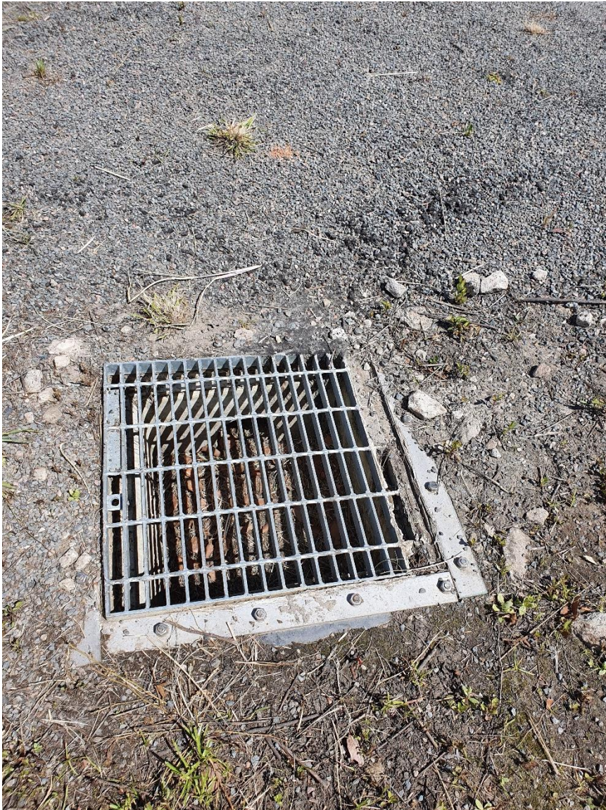
Figure F7. Stormwater drain pits require cleaning.
