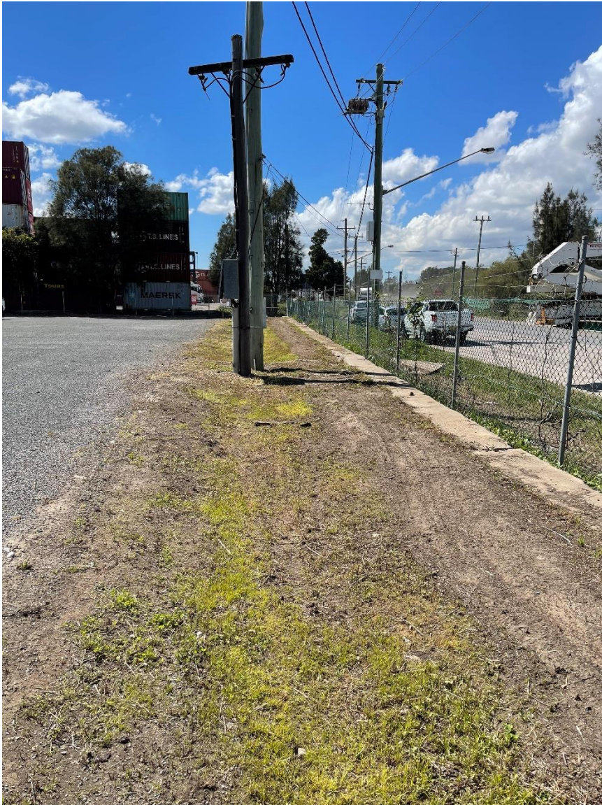
Figure F3. Grass drainage swale along the front boundary of the site.
